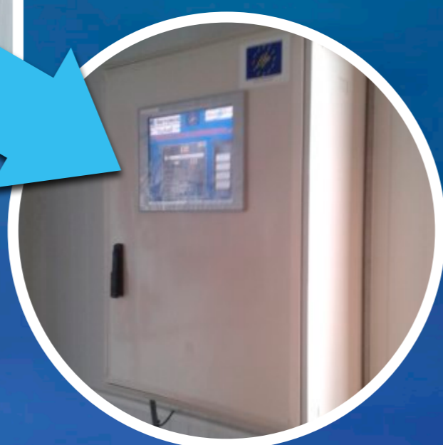
Programmable Logic Controller (PLC)
